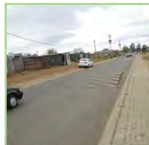
Picture 29: Vegetation growth on sidewalk
