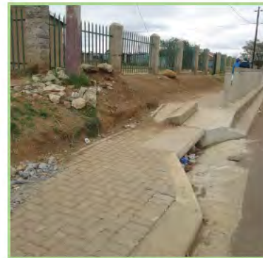
Picture 23: Blocked kerb inlet
