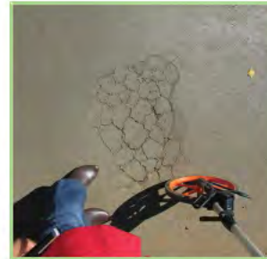
Picture 20: Sign of distress
