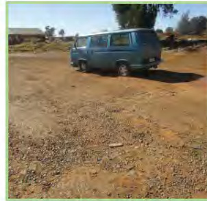
Picture 35: Poor grading and finishing
