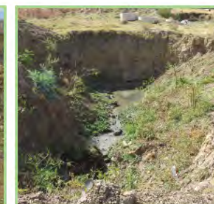
Picture 32: Raw sewage flowing from the existing sewer line
