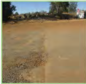
Picture 34: Poor construction of surface joint
