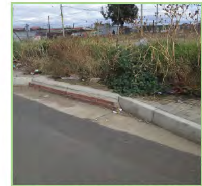
Picture 24: Closed kerb inlet
