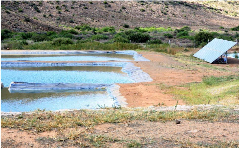
Above: A part of the first phase of the wastewater works project in Nieu Bethesda has been completed.
