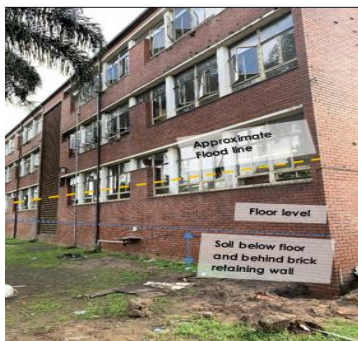
School classrooms structurally unsafe for use
