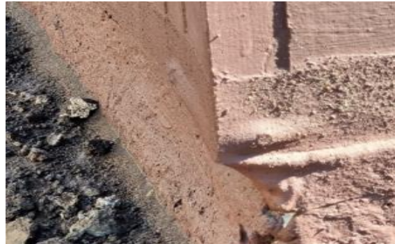
Wall panels positioned outside concrete slab's edge
