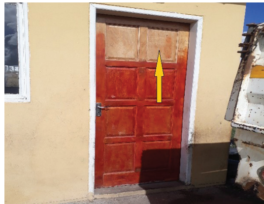
Door not fully painted
