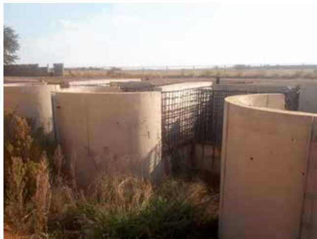
Reinforcing steel severely affected by rust
