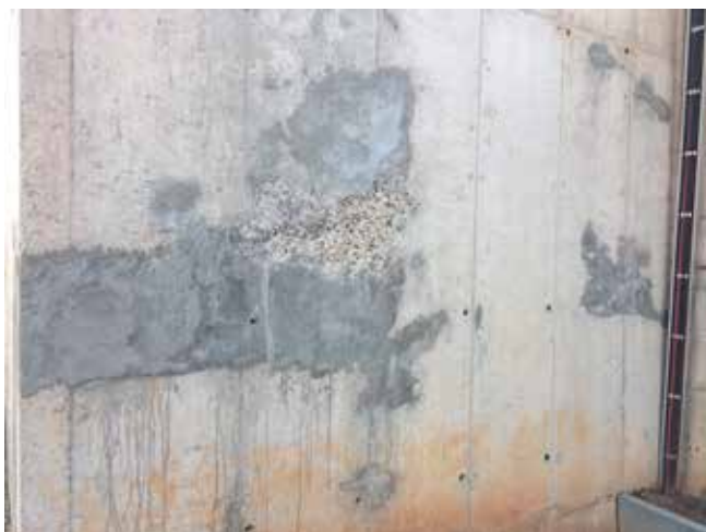
Poor concrete work
