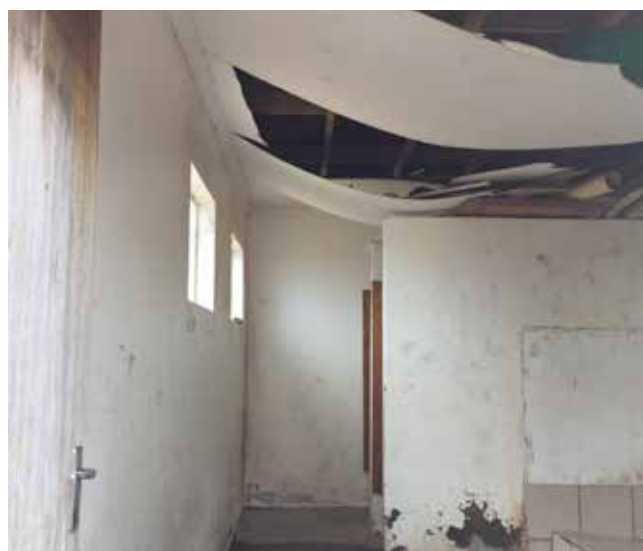
Blocked toilets and ceiling close to collapsing
