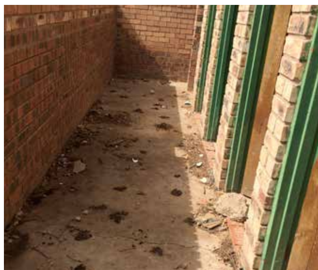
New toilets not connected to reticulation system
