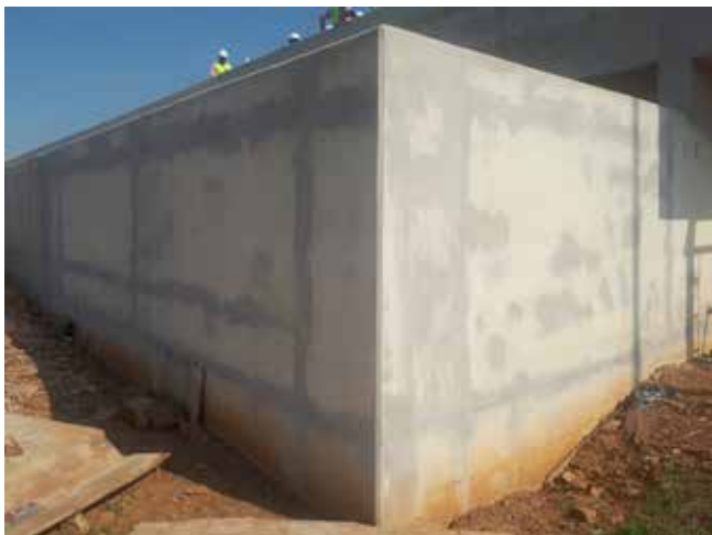
Lots of patched cracks on concrete
