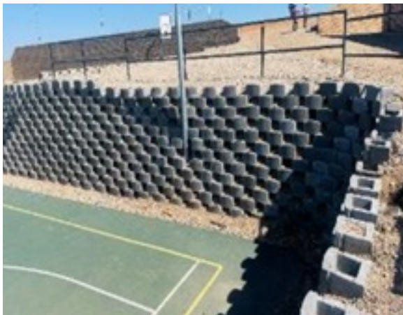
Top retaining wall blocks loose
