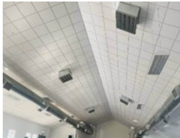
Leaks around ventilation units due to poor waterproofing
